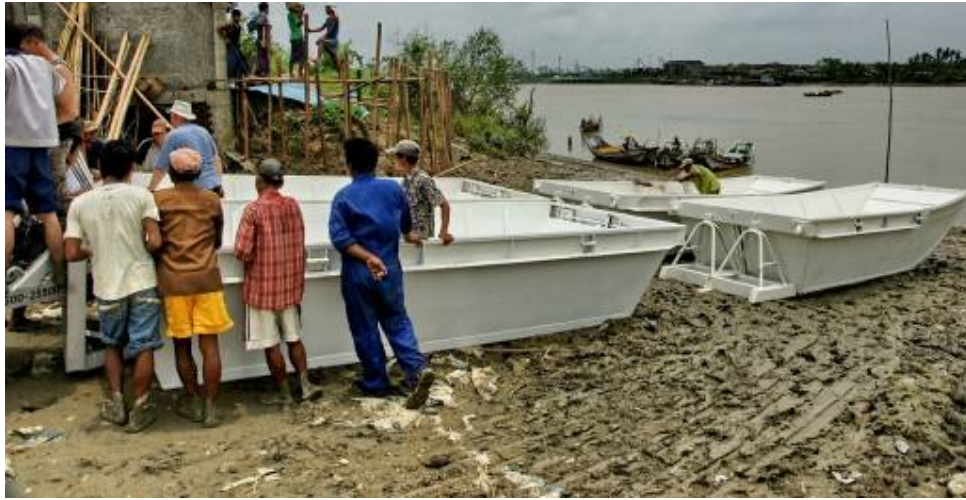
Assembling the river boats beside the Hlaing River - The assembly connection points can be seen clearly between the two halves of the aluminium hulls, with the Hlaing River in the background - 19 th May 2008
