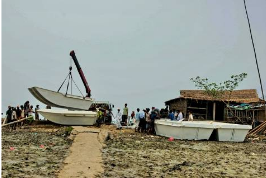
Unloading the boats by crane at the Hlaing River outside Yangon ready for assembly beside the Hlaing River by a team under the supervision of UK experts - Monday morning, 19 th May 2008
